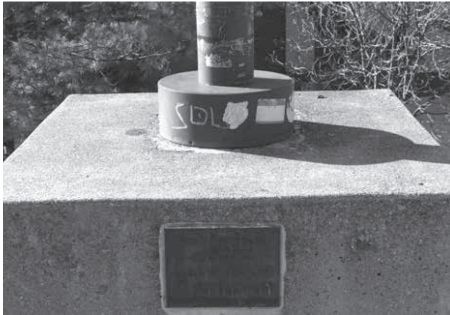
Figure 3: SOL on a Lamppost South of the College Avenue Bridge
